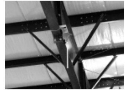
MACDAC Wireless LAN Communications: Wireless access point on Stowe Machine's wired eXtremeDNC™ server network communicates with wireless Ethernet adapter mounted at the machine tool.
