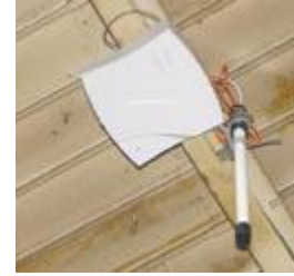
The wireless access point and antenna are mounted to the ceiling above a machining area. The access point is wired to the DNC server and is powered without a separate electrical line.
